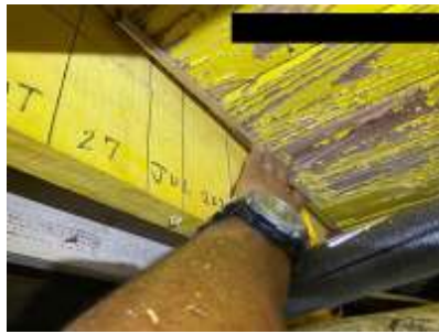
Two Nails per Board #2
