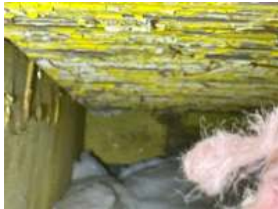
Metal Connectors #2 (3 Nails Noted)
