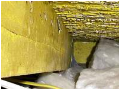
Metal Connectors #1 (3 Nails Noted)
