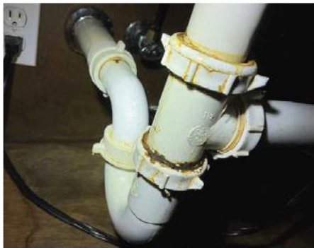
Worn out plumbing lines
