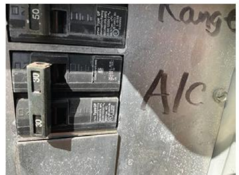
Installed circuit breaker
