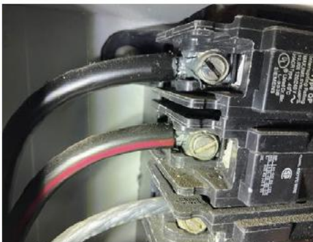
Multi-strand aluminum wiring-acceptable
