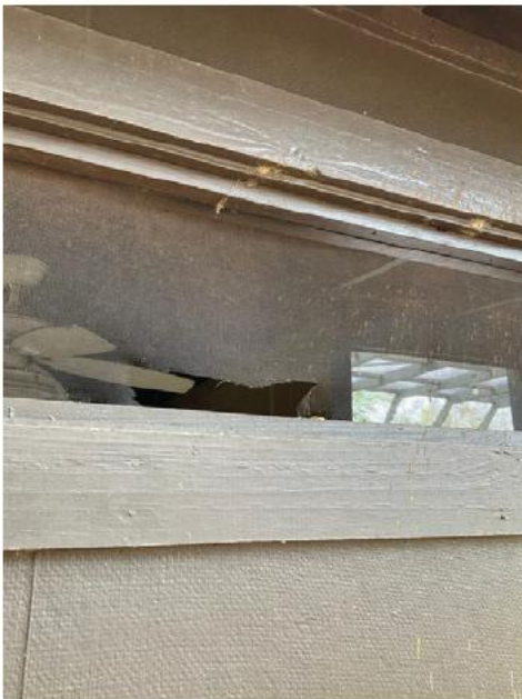
Damage screens/various areas
