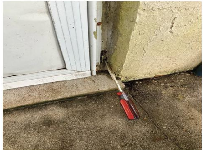
Wood Decay Front Door Frame Right
