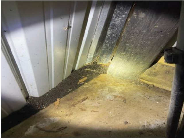
Wood Decay Detached Garage Perimeter/Various Areas
