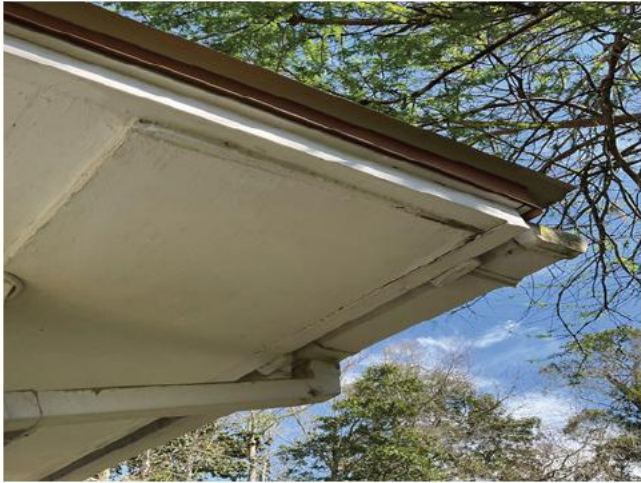
Wood Decay Right Side Eave Near Rear
