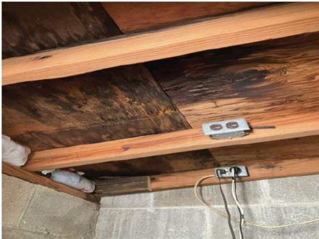
Wood Decay Well House Roof Sheathing
