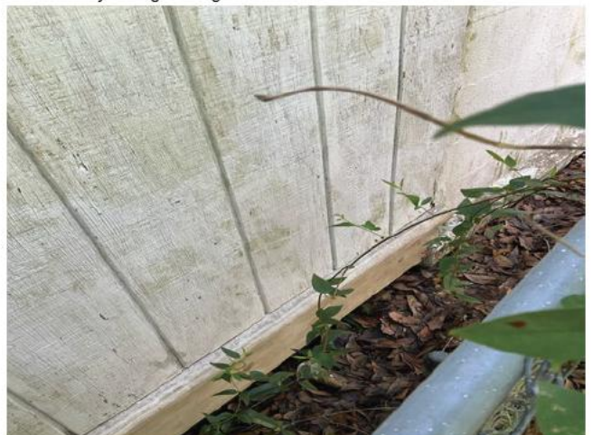
Wood Decay Cottage Siding Rear/Lower Half/Various Areas
