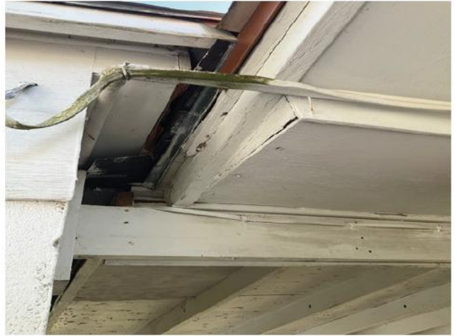
Wood Decay Rear Eave/Cottage And Main Connection
