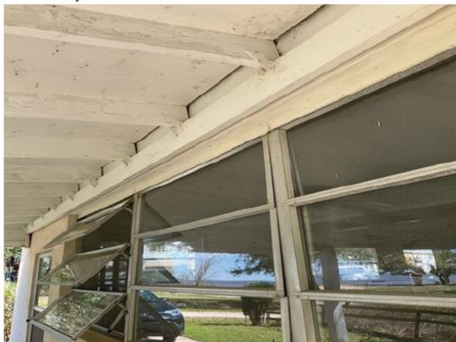
Wood Decay Right Side Window Frame/Upper Half/Various Areas
