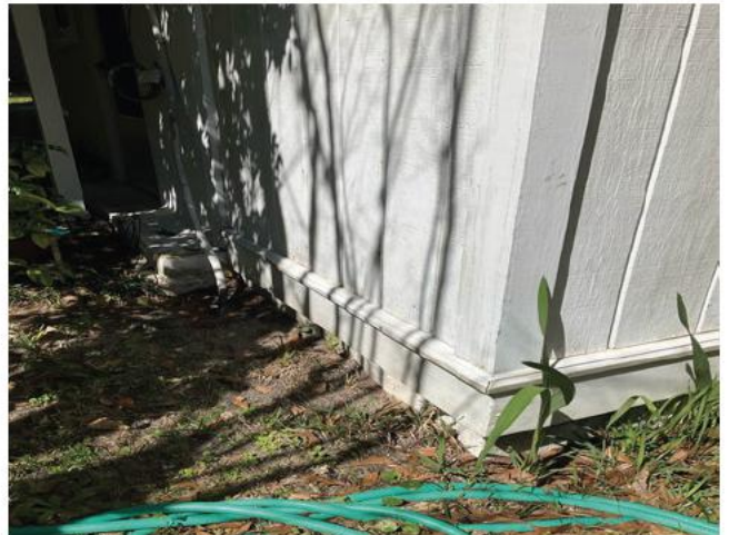
Wood Decay Cottage Siding Front/Lower Half/Various Areas
