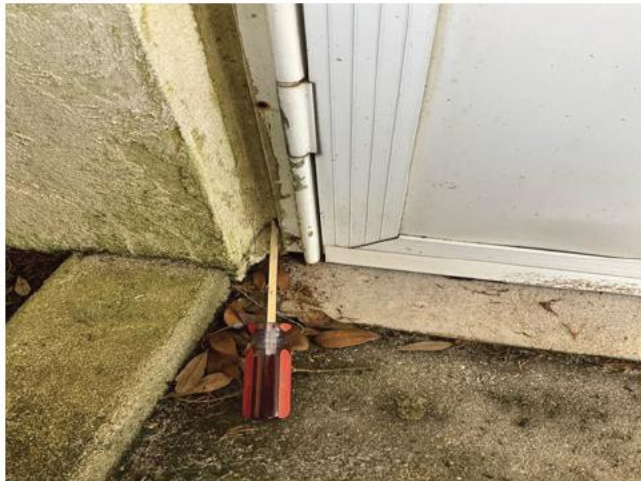
Wood Decay Front Door Frame Left
