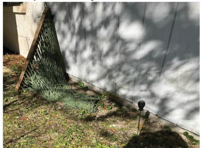
Wood Decay Right Side Siding/Lower Half/Various Areas
