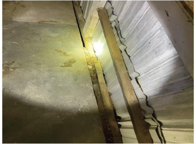
Inspection Limited/Earth To Wood Contact/Detached Garage Perimeter
