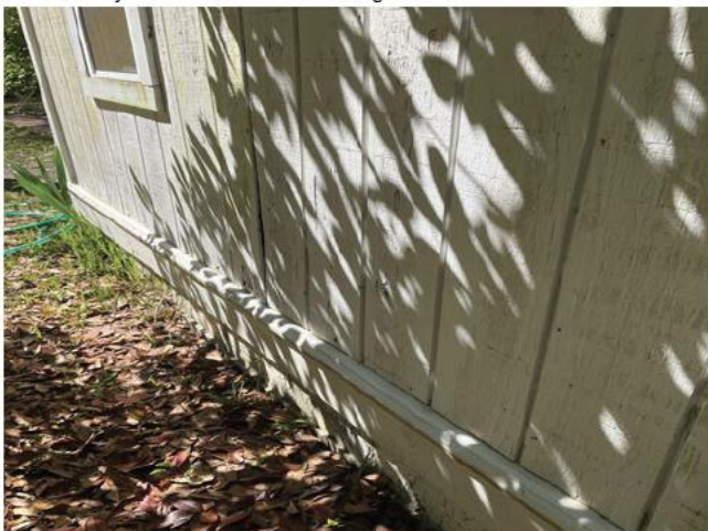
Wood Decay Cottage Siding Right Side/Lower Half/Various Areas
