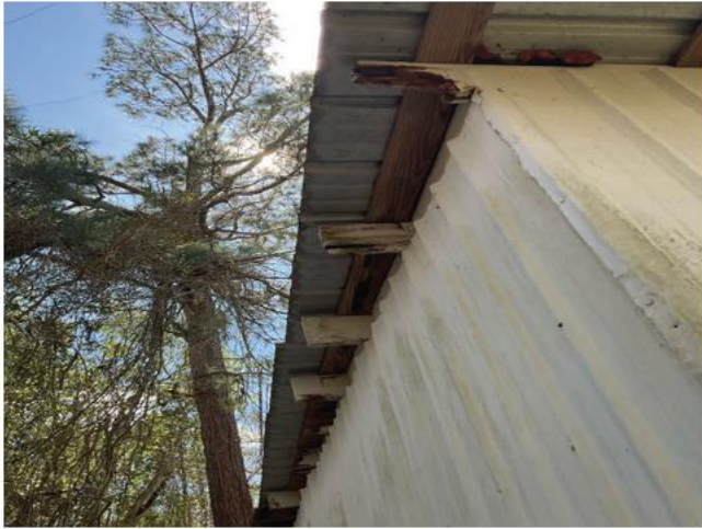
Detached Garage Rear Rafters/Eave At Various Areas
