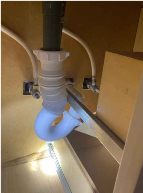
Improper drain pipe installation/missing shut off valves
