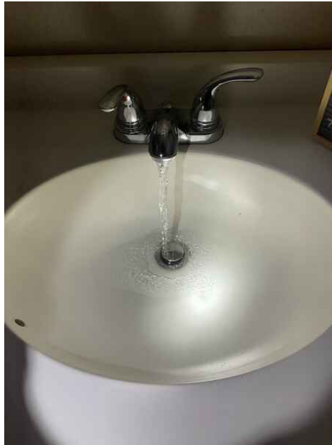
Drain Stop Inoperable
